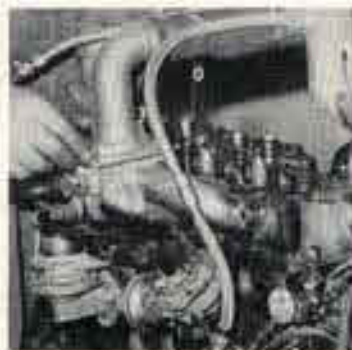
Manifold pipe, fuel pipe and oil supply connections.
