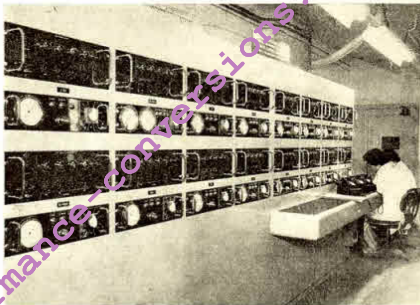
The control panel of the automatic liquid-metering system designed by Automatic Control Engineering Ltd. for General and Industrial Paints Ltd.
